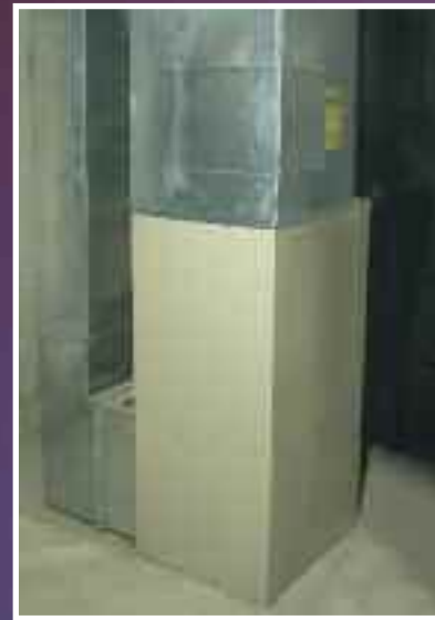
Hydro-air and heat pump backup
